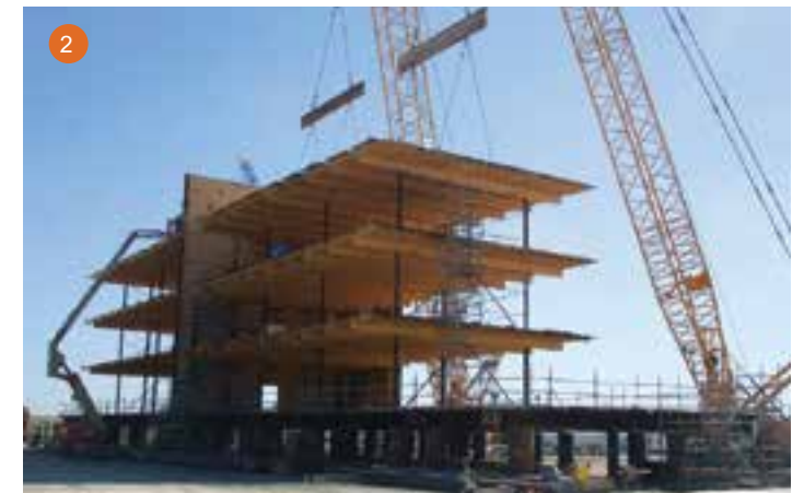
1. Crews continue fabrication of a 4,500-ton drill rig topsides destined for the Gulf of Mexico. 2. KOS teamed with Kiewit Building Group to construct the 192-man living quarters for a 25,000-ton topsides. Both the living quarters and the topsides are being built at the KOS yard.
