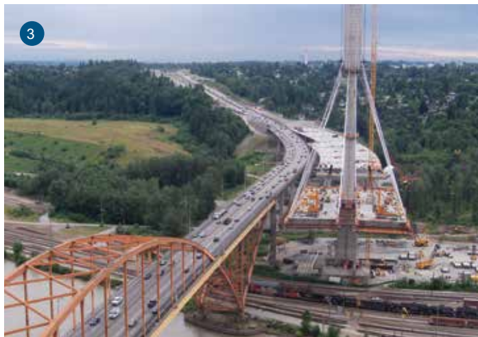
1. The “structures gang” celebrates a job well done at the new Port Mann Bridge. 2. Segment 4 of the project includes the widening and upgrading of miles of Highway 1 as it winds throughout Surrey, a suburb of Vancouver. 3. The new Port Mann Bridge goes in alongside the old bridge, which opened in 1964. The old bridge will be torn down when the new version is completely finished and opened to traffic.
