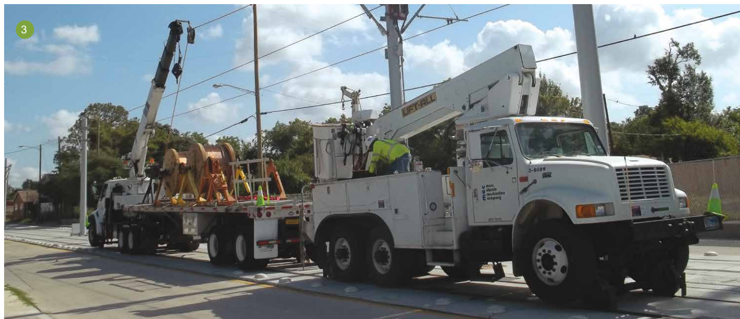
1. This platform truck is ideal for two-person operations. The scope of MEC’s work includes more than 16 miles of overhead catenary, consisting of nearly 1,000 OCS poles, 1,500 cantilevers and 455,000 linear feet of overhead wire. 2. MEC’s custom-built bucket truck with integrated regulating arms makes overhead contact systems work safer for the crew. 3. MEC’s wire-stringing operation requires significant planning and preparation to ensure excellent execution.
