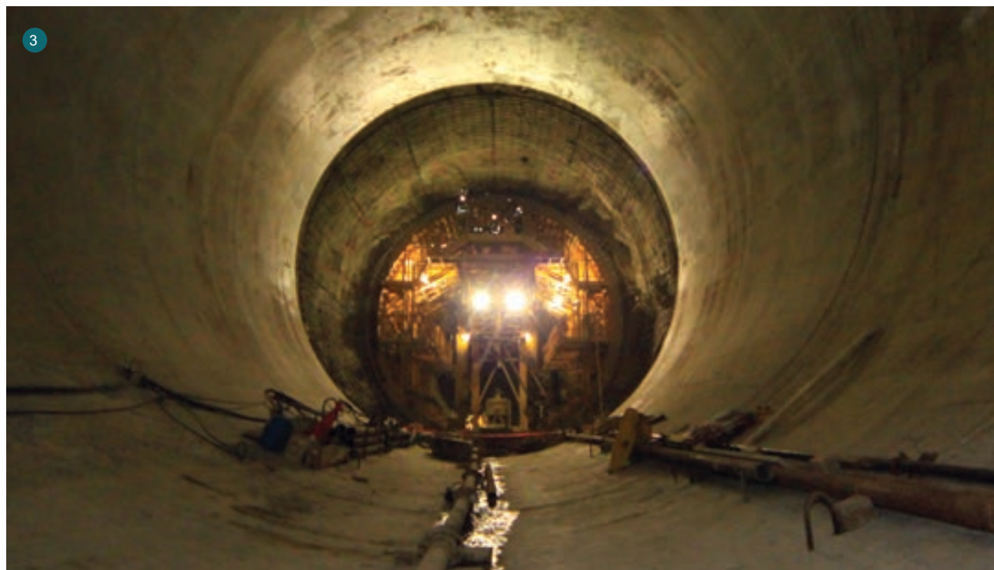
1. Kiewit employees lower and raise tools to each other while working on the concrete tunnel finisher. 2. Maria Garcia prepares to radio workers on the surface to lower the heavy equipment 300 feet down into the tunnel. 3. A wide-angle shot of the concrete finisher from the inside of the McCook Tunnel.
