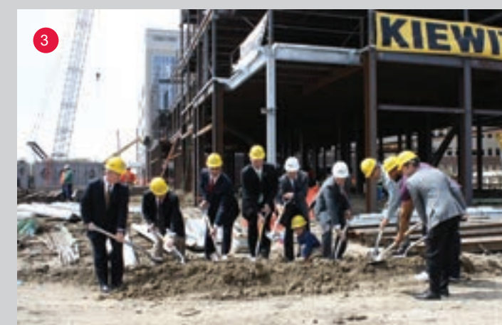
1. Kiewit employees and subcontractors gather for a mass safety meeting. 2. Canopy Street hotel and condos view from corner of ‘Q’ & Canopy Streets. 3. Developers, city officials and Suh break ground on the Hyatt Place hotel and Hobson Place in April 2013.
