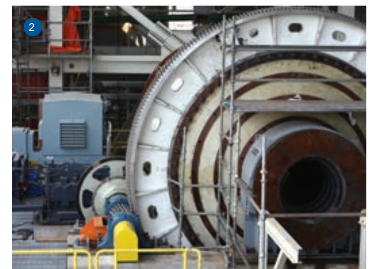
1. The La Cygne generating station is home to this Flue Gas Desulphurization building and its massive maintenance alley, which measures 300 feet long. 2. As part of the limestone slurry preparation area, millwrights erected and aligned two ball mills (pictured). Once in operation, each is capable of producing up to 66 tons of slurry per hour.
