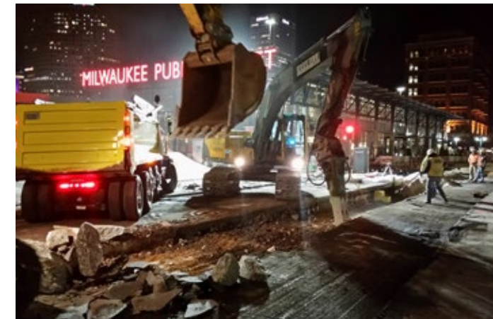
Excavation through critical intersections was often performed on nights and weekends to minimize disruption to traffic.
