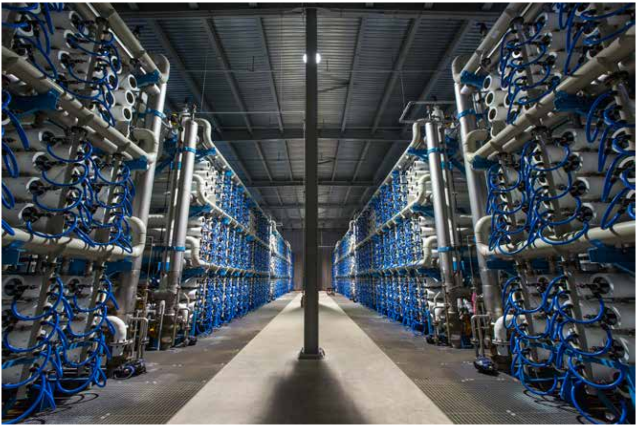
The project team for construction of the Carlsbad Desalination Plant used a three-dimensional model to design the plant's reverse-osmosis building and consequently could ensure adequate spacing and safe access to machinery and instruments. Photo courtesy of Poseidon Water
