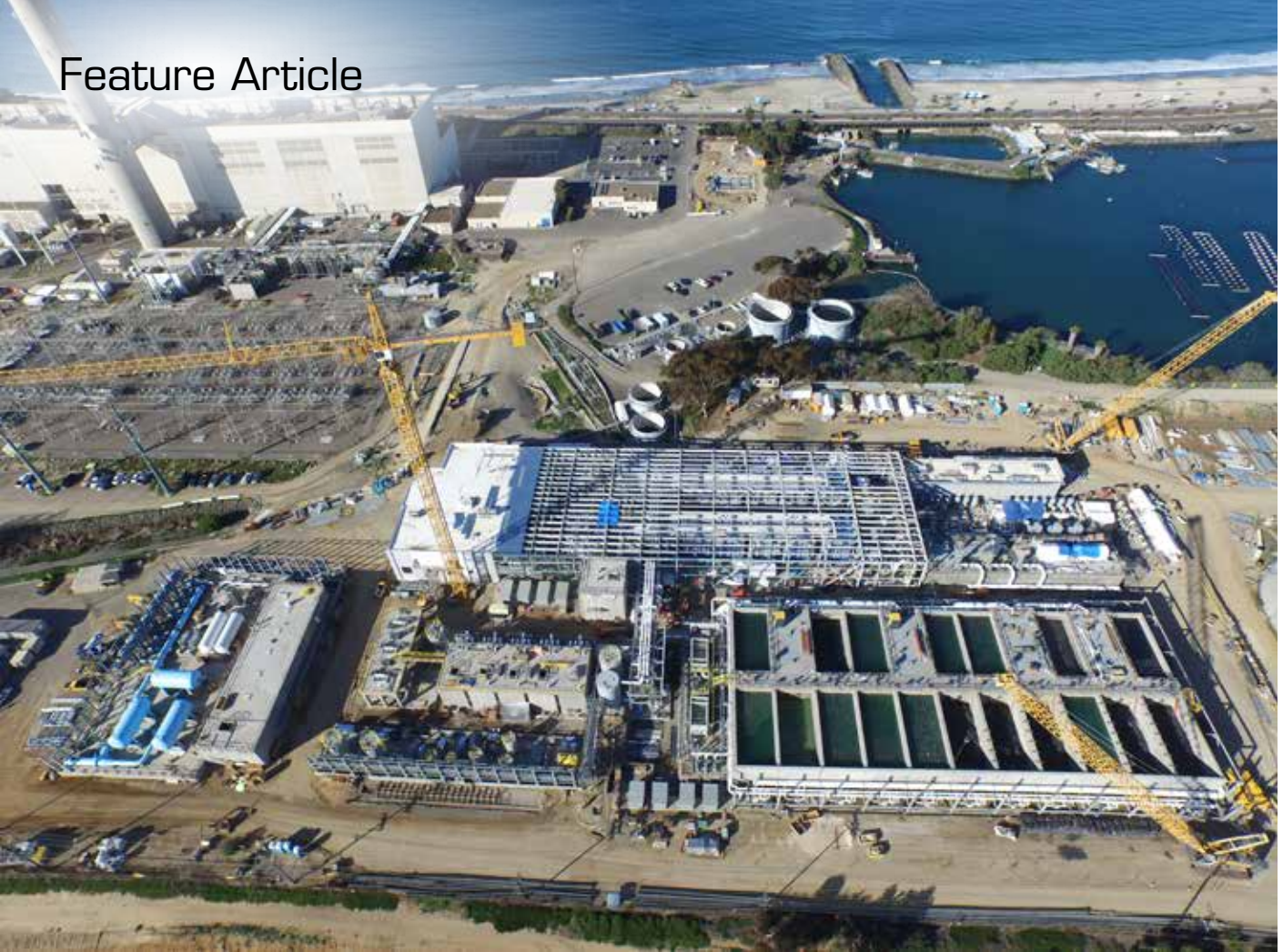
A sound communication plan contributed to the success of the Claude “Bud” Lewis Carlsbad Desalination Plant project in Carlsbad, Calif., which used a design–build–operate model. Image courtesy of Poseidon Water.
