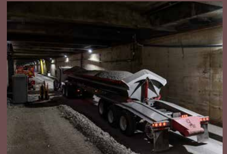
Kiewit used recycled viaduct material as an environmentally friendly solution to fill the decommissioned Battery Street tunnel. Photo credit: Washington Department of Transportation
