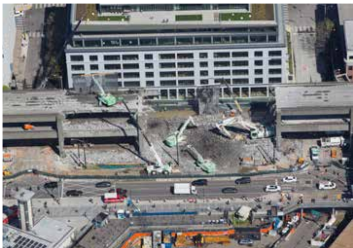
These photos show just how close the viaduct was to buildings and nearby surface streets, making it more critical that the project team mitigate the effects of vibration, noise and dust.
