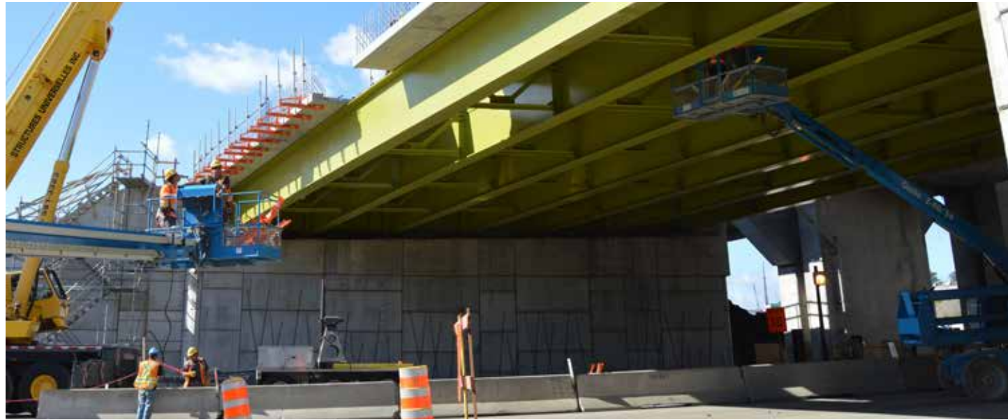
Girders, guardrails and retaining walls were painted green in this neighborhood to blend into its urban décor. Other neighborhoods were painted red, blue, yellow and gray.
