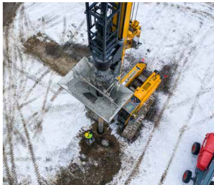
Kiewit Foundations installed 1,022 non-vibratory stone columns at the new Kiewit Headquarters in Omaha, Nebraska. Each is 24 inches in diameter with a depth ranging from 20 to 30 feet. Kiewit is the only contractor that has installed non-vibratory stone columns in North America.
