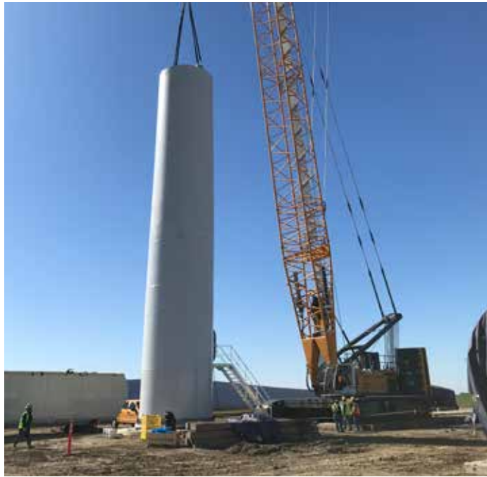
The base section of a wind turbine is set at Timber Road IV. Each wind turbine has five to six tower sections.
