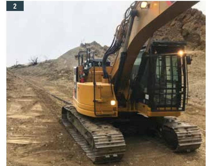
1. A CAT 325 excavator makes its way down a 70% grade slope tethered to a Falcon winch assist machine. 2. The tethered excavator.
