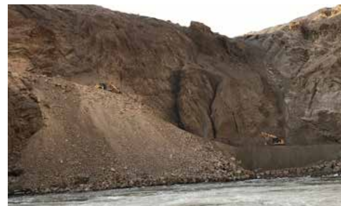
This excavator was used to build the toe of the embankment to minimize material loss in the river as trucks dumped blast rock from the top of the slope.
