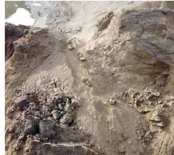
Crews drill, excavate and work on embanking the access road in the through cut.
