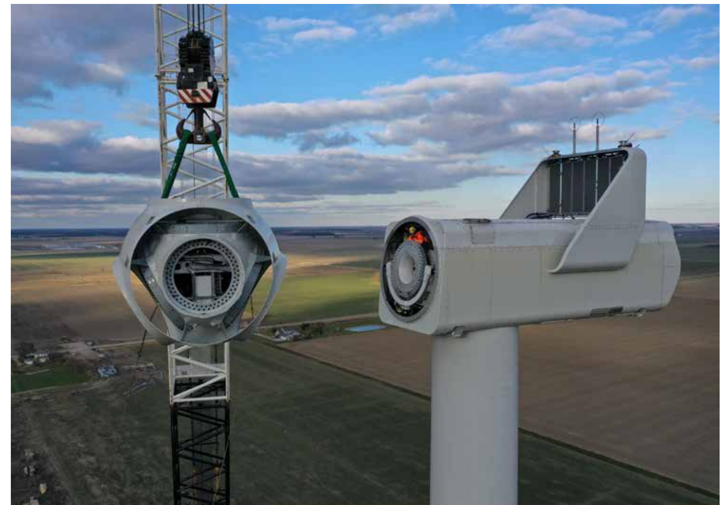
The hub of this Vestas V150-4.2 megawatt turbine is shown being set on the nacelle. The blades will be attached to the hub, which is 105 meters high.
