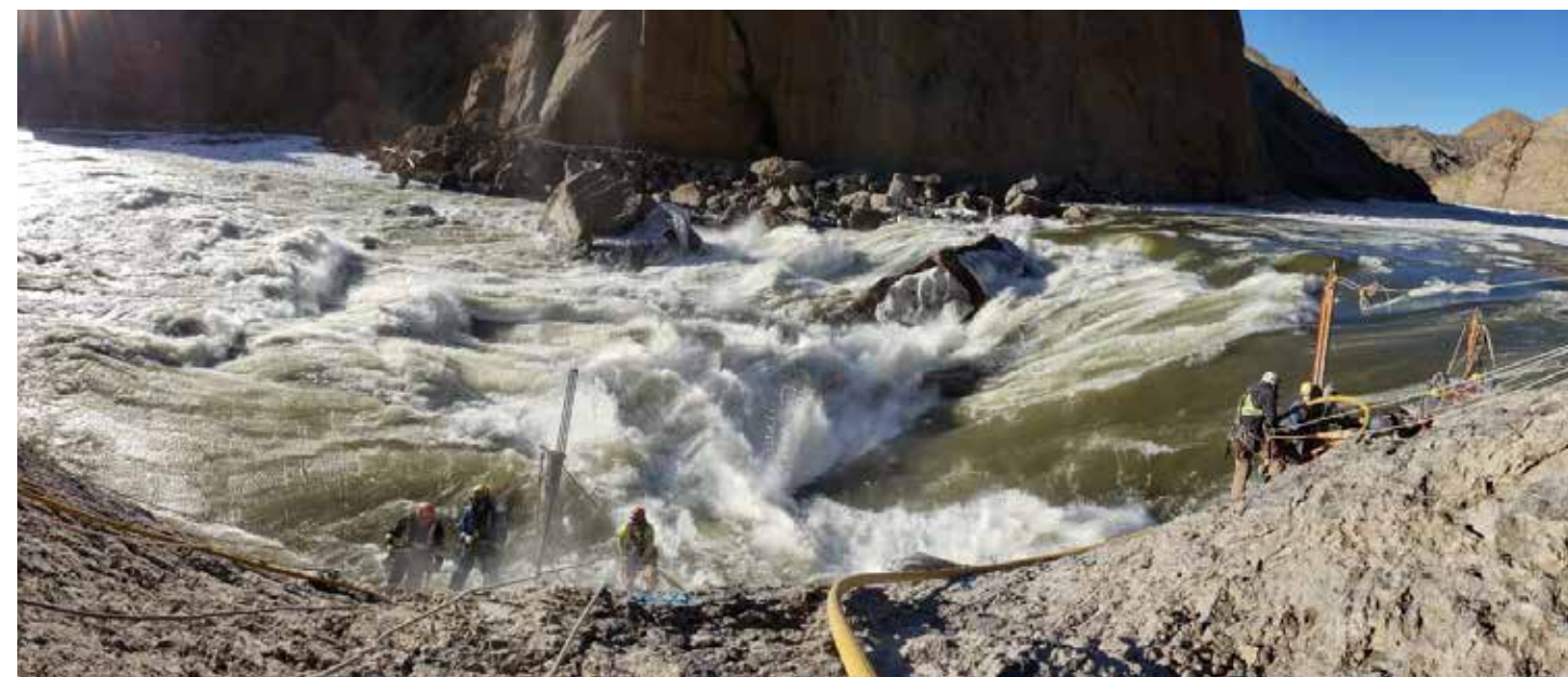
Crews drill blast holes on the East Toe for channel constriction widening.
