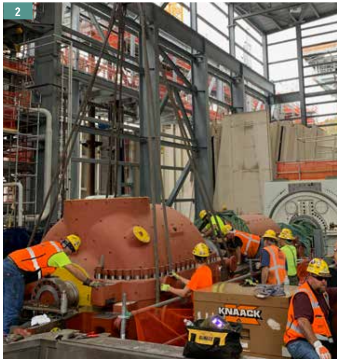
1. GE's Alstom Heat Recovery Steam Generator. 2. The millwright crew sets up the IP Turbine. 3. This photo captures the final touch-down of the generator. 4. Kiewit's new Liebherr 11000 crane is used to set a pipe rack module.
