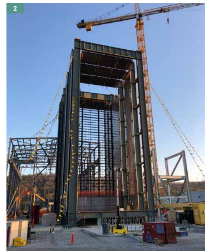
1. Cable pull operations are set up along the cooling tower. 2. The Heat Recovery Steam Generator casing is shown near completion.
