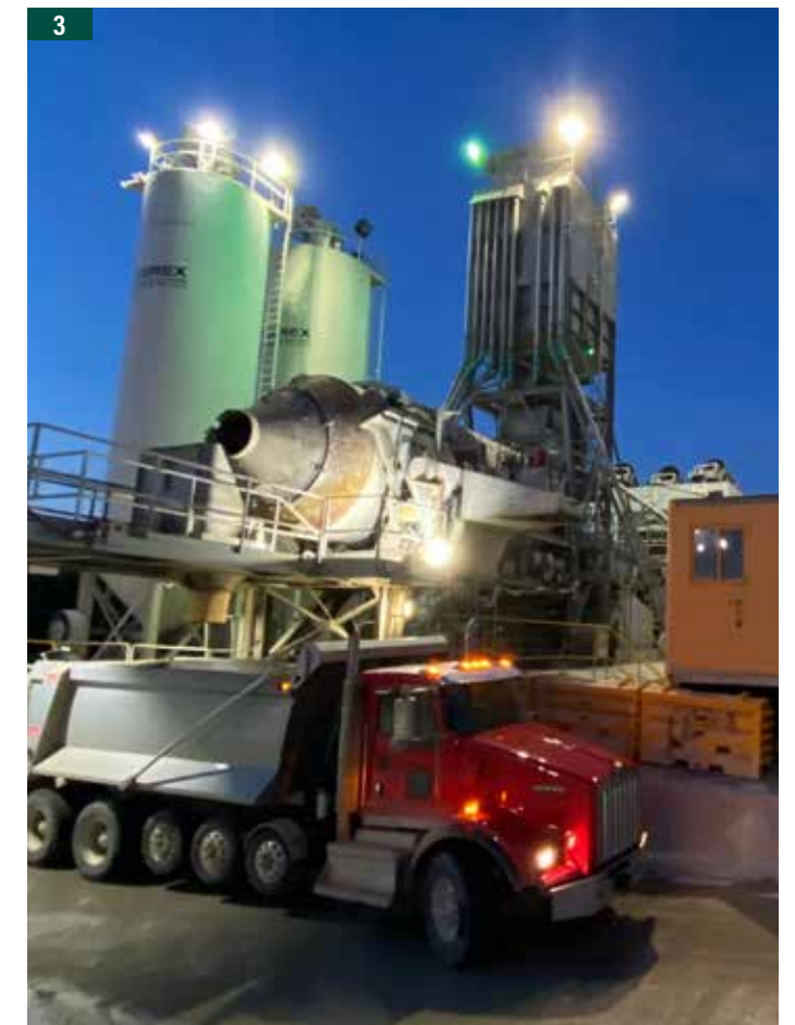
1. Crews perform 13-inch slip form paving on State Highway 121 using a GNZ600S slip form paver. 2. Northbound State Highway 121 Collector Distributor deck pour. 3. Aggregate is processed on-site at the NorthGate Constructors batch plant.
