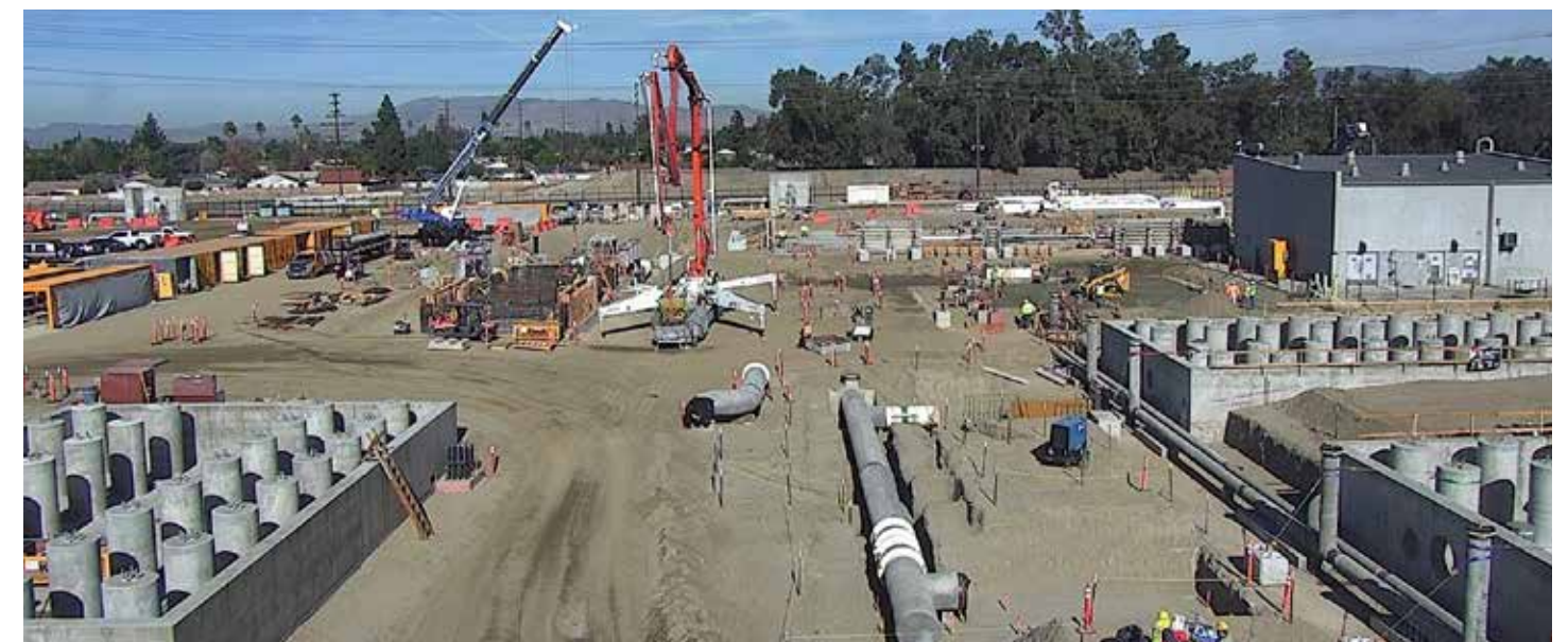
Crews install underground piping and electrical systems in addition to the granular activated carbon (GAC) vessel support columns (shown in the foreground) on the Tujunga site. The North Hollywood and Tujunga plants will extract water from two sets of existing, non-producing groundwater wells, treating 50 million gallons a day and 25 million gallons a day, respectively.
