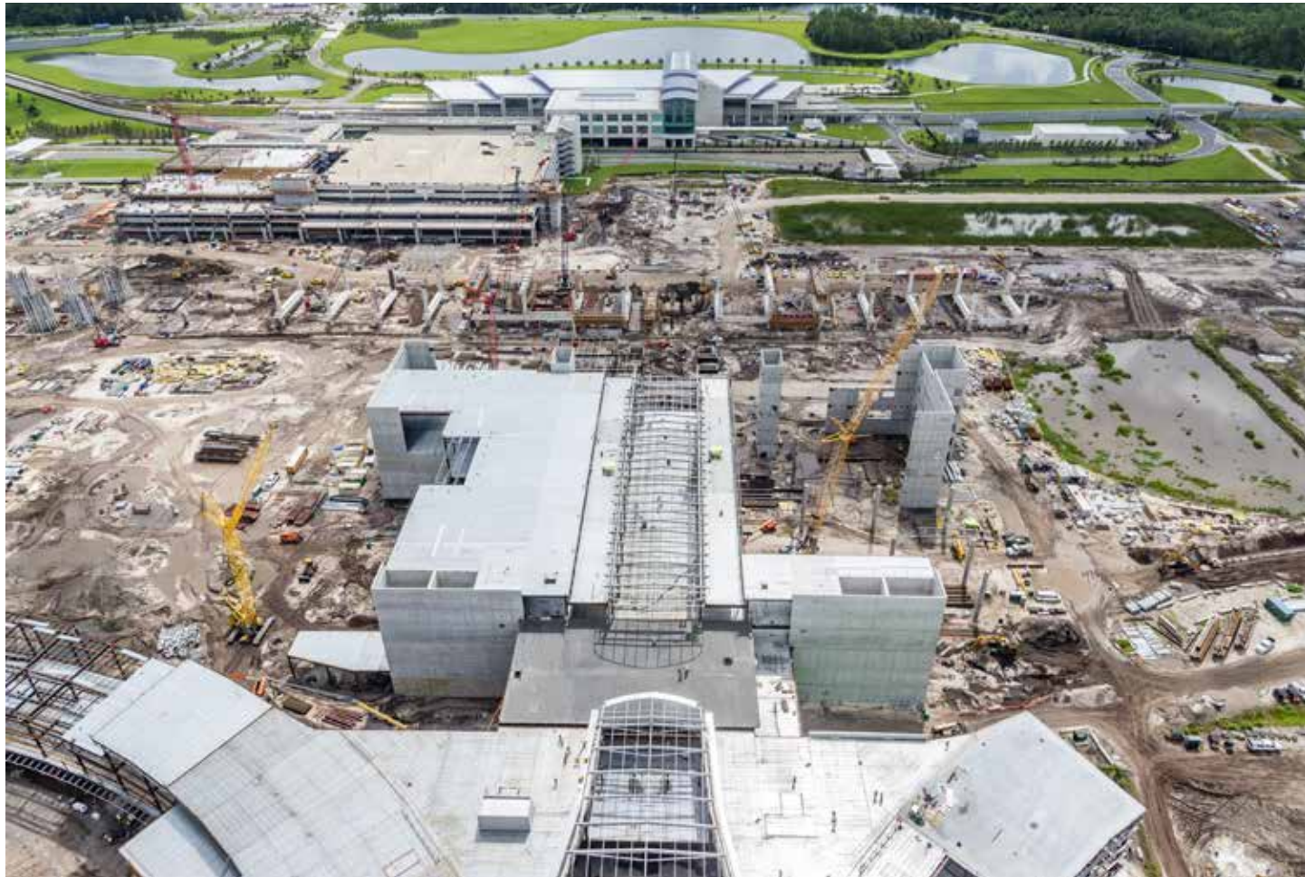
Kiewit shared the project worksite with more than 90 contractors and subcontractors, making daily coordination critical to meeting access and space needs. All parties worked together to ensure everyone had safe access to their parts of the program.
