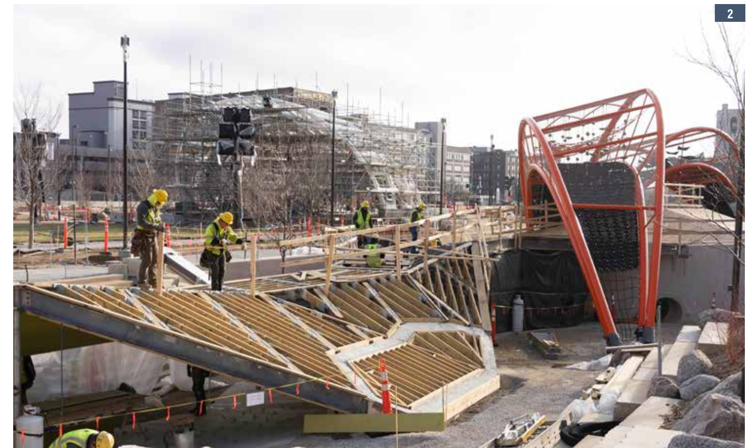
1. Gene Leahy Mall, reopening summer 2022, features a Sculpture Garden, Arches Playground, Performance Pavilion and more. 2. Crews constructed Arches Playground with extra special areas for kids to explore, including a climbing wall, rope forest and plenty of shade for the hot summer months.
