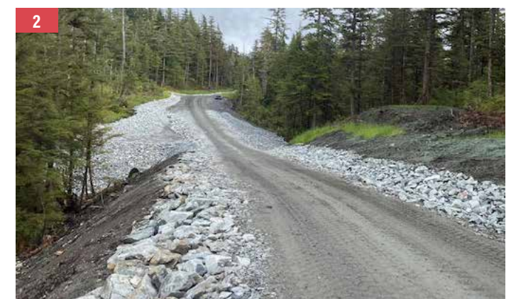
1. Crews assembled the multi plate on site in 4-foot sections due to access and transport limitations. 2. The road was constructed with materials obtained through the excavation and drill and blast process.
