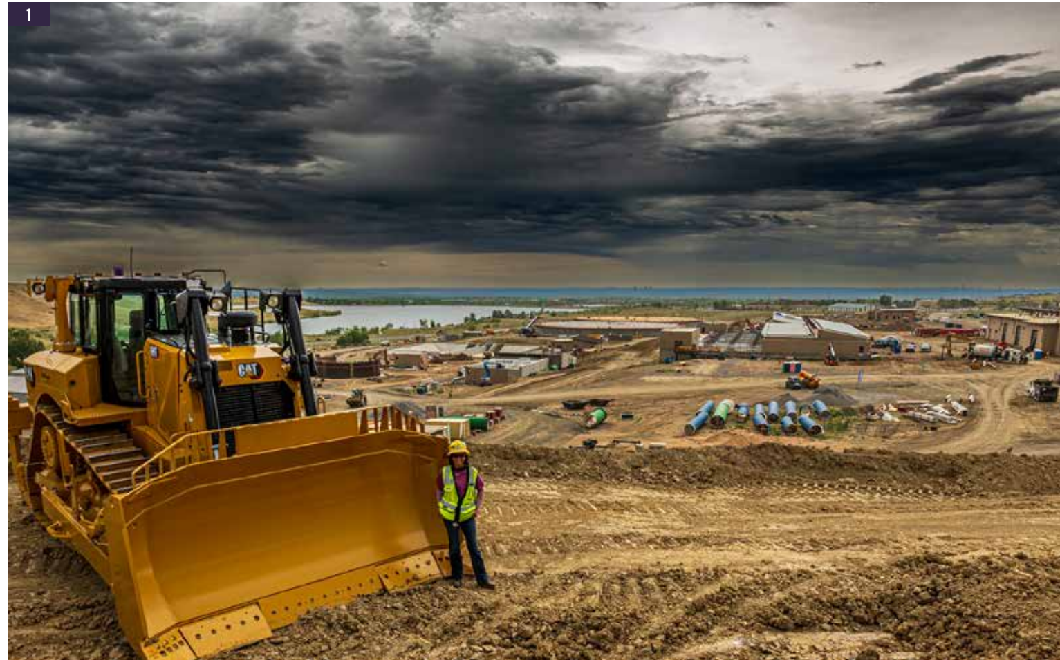
1. Sanchez pictured next to a D8 dozer on the job site in Golden, Colorado. 2. Blount standing on the deck of the D.B. Alameda, the derrick used on-site.
