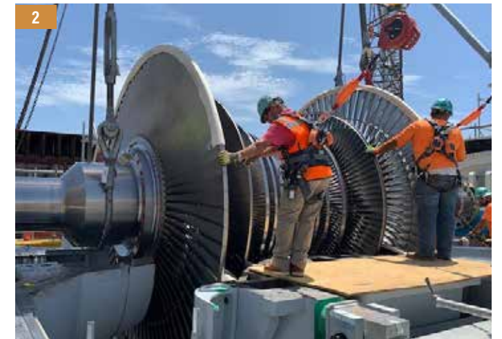
1. In total, the team carefully assembled and placed approximately 8,700 tons of equipment, including the turbines, generators, steam drums, transformers and HRSG modules. 2. The project team sets in place a turbine guided by a 716-ton crane.
