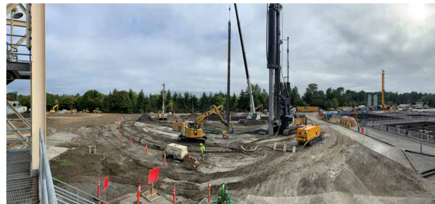
Ground improvement techniques, such as deep soil mixing and jet grouting, prepared the soil to ensure new structures were stabilized and met updated seismic standards in the event of an earthquake.
