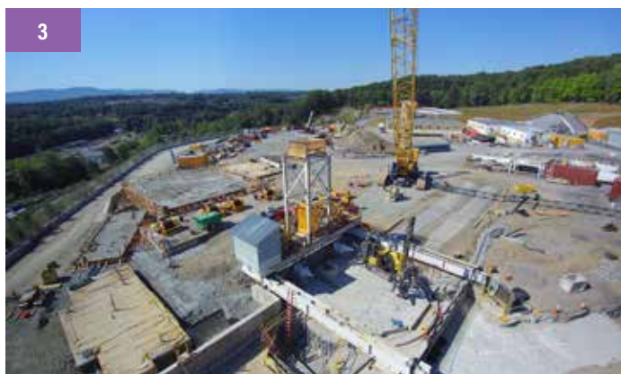
1. The shaft mining site with the signature "head frame" over the shaft also included storage for the precast tunnel lining. 2. The underground chamber being prepared for the assembly of the TBM. 3. Foundations being placed for the buildings housing the hoists that service the shaft.
