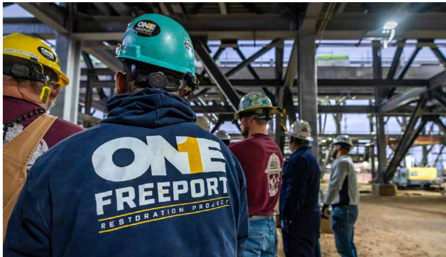
The foremen's meeting on the Freeport LNG project was an interactive experience each week. The typical meeting was revitalized using the Front-Line Supervisor (FLS) Safety Leadership training and development manual. The focus was not only on safety, but also developing leaders who understand the safety culture and can lead the business into the future.
