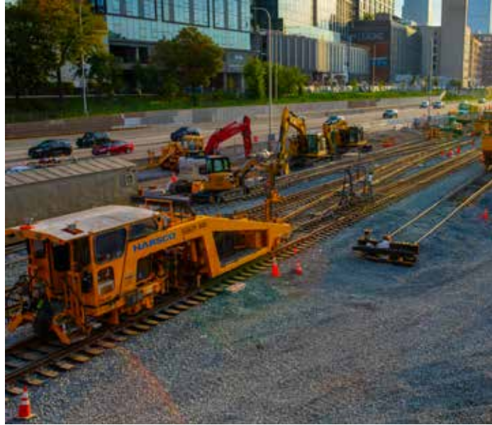
A tamping machine is used to align and compact the ballast underneath the railroad ties, keeping commuters' rides smooth.
