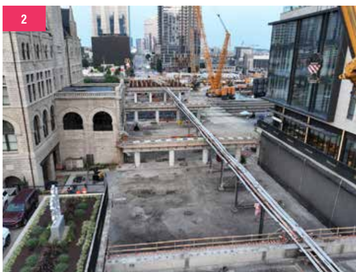
1. Kiewit used precast concrete panels for the deck as part of the accelerated bridge construction process. The bridge was raised about two feet over the railroad to meet new construction standards. 2. Kiewit meticulously disassembled the original bridge to preserve the existing AT&T fiber-optic lines and maintained uninterrupted service to the downtown area.
