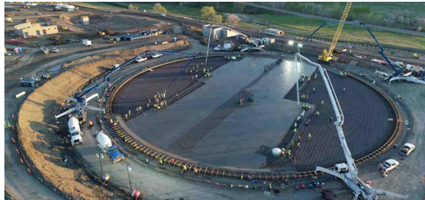
Kiewit's in-house team delivered expertise when the initial concrete pours needed adjustment, creating and testing a new mix in just a few weeks. The pour pictured above was performed by subcontractor Garney Construction.
