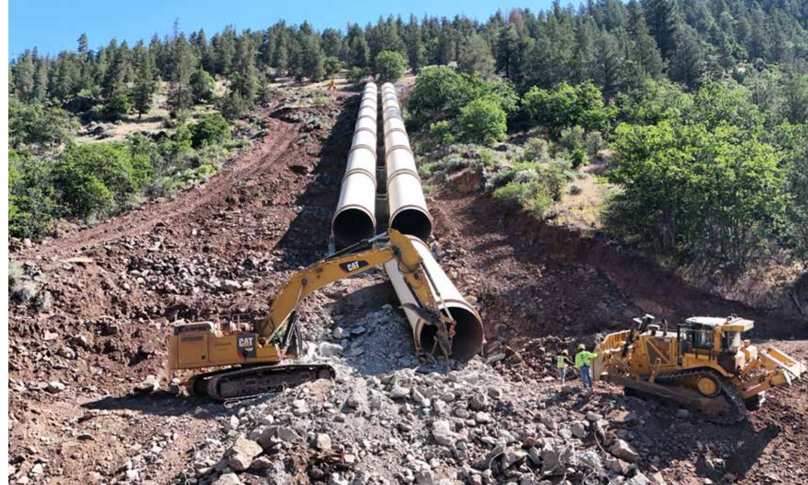
One of the most challenging aspects of demolishing the JC Boyle earthen dam in Oregon was the removal of double penstocks, each about 10 feet in diameter. Water was kept level for about two miles, then dropped down the steep mountain in penstocks to drive power. The team brought in track line excavators to reel equipment down the steep slopes.
