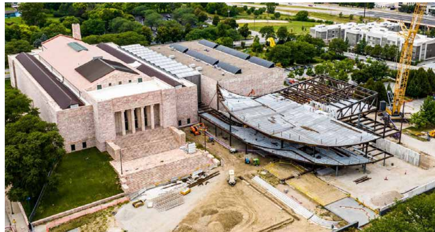
The new Rhonda and Howard Hawks Pavilion, shown under construction in the photo above, required a complex steel structure, including large cantilevers that extend 40 feet out and above the main level of the building. Its curves are in stark contrast to the original rectangular museum buildings.
